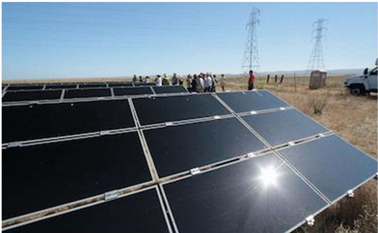
Figure 11: Typical PV module arrangement in N-facing frame, with variable tilt about the E-W axis
